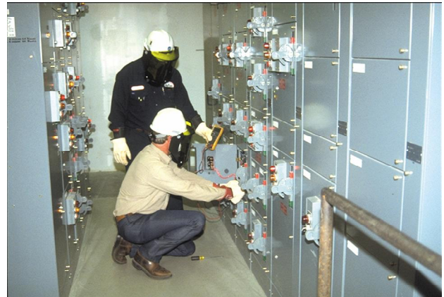
Figure 7 Flash Hazard Analysis Determines the Level of Protection Required on this Motor Control Center (Category 2, 8 cal/cm 2 )
